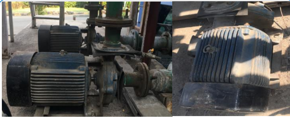
Before- KDI-1000 type, 7.5 HP two IE1 class induction motors are working for cooling tower water circulation.
